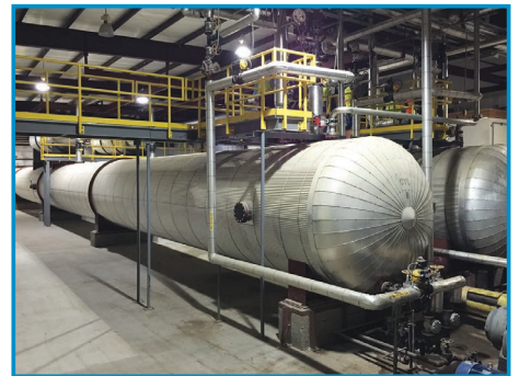
This treating plant is set up with two cylinders and is a dedicated railroad plant treating with creosote and borates.
