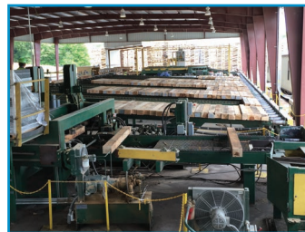
This view is of the plating and sorting portion of the operations.
